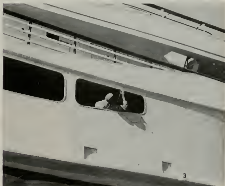
Fig. 3—Spray painting will enable the yard to launch this boat days sooner than if hand brushing were used. Most surfaces of the boat are painted with this type of air-operated equipment.
